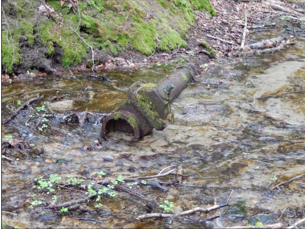
Figure 39. Steel pipe and valve near the location of the former fish hatchery.
