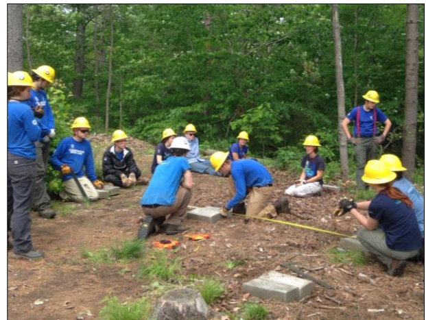
Starting foundation on camping shelter during training at White Lake State Park
