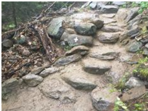
Rock staircase constructed on the White Cross Trail during one of five hitches at Monadnock SP.
