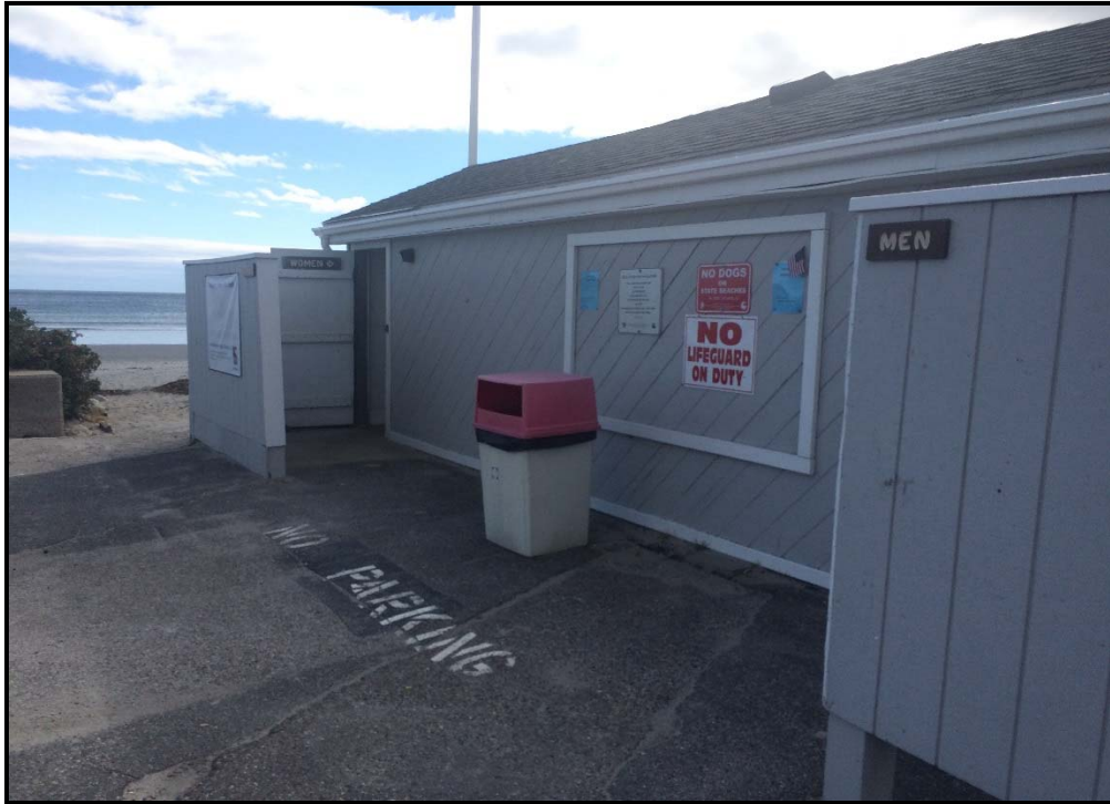
Photo 5: View southeast at the existing Jenness State Beach bath house. The existing bath house will be replaced with a larger structure that will be relocated immediately north of the existing structure within the existing parking lot.
