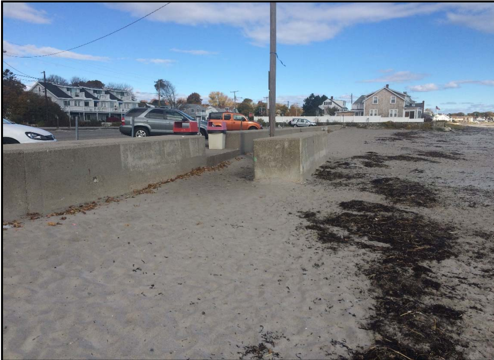
Photo 4: View north along the existing concrete seawall which denotes the eastern boundary of the project area.
