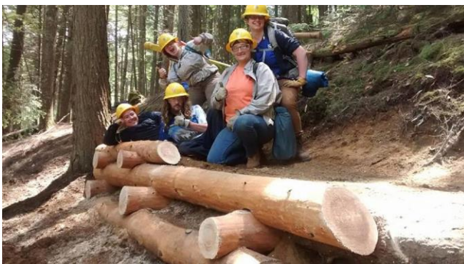
Native hemlock retaining wall constructed during Trail Work Skills Training, Hemlock Trail, Bear Brook SP
