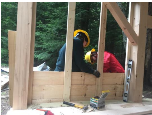
Attaching waney-edge siding on a camping shelter during training at Crawford Notch SP
