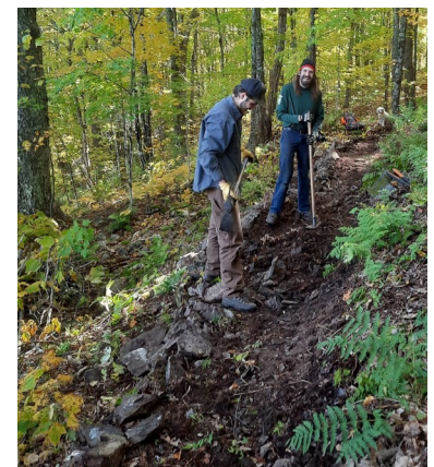
WSPA and TCTA constructing a new loop trail at Weeks State Park.
