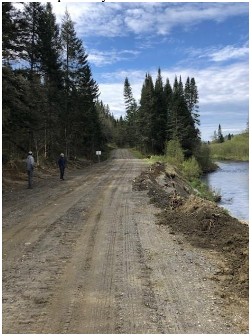
Figure 2- Shows the washing on Indian Stream Road
