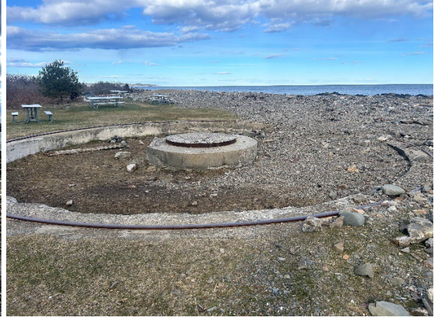
Needs to be cleaned out to grade
